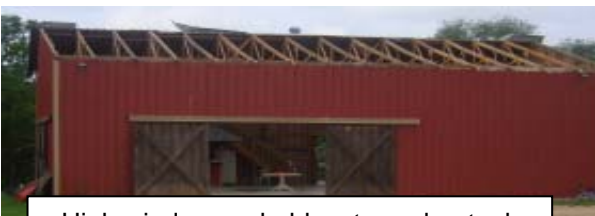
High winds – probably a tornado - took the roof off of our barn at River Ranch. No one got hurt.
